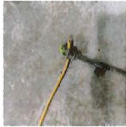
extension cord wired into the two ends of a service cord
