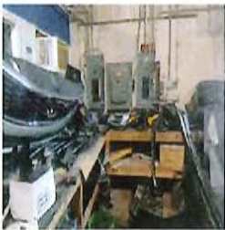
blocked electrical panels
