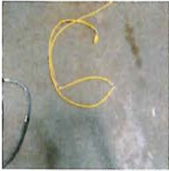
extension cord in bad shape in shop
