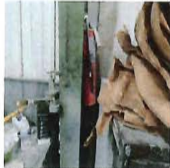
blocked fire extinguisher in shop
