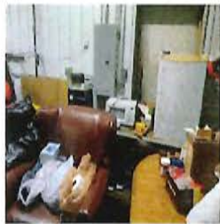
blocked electrical panel
