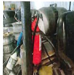
service extinguisher on forklift
