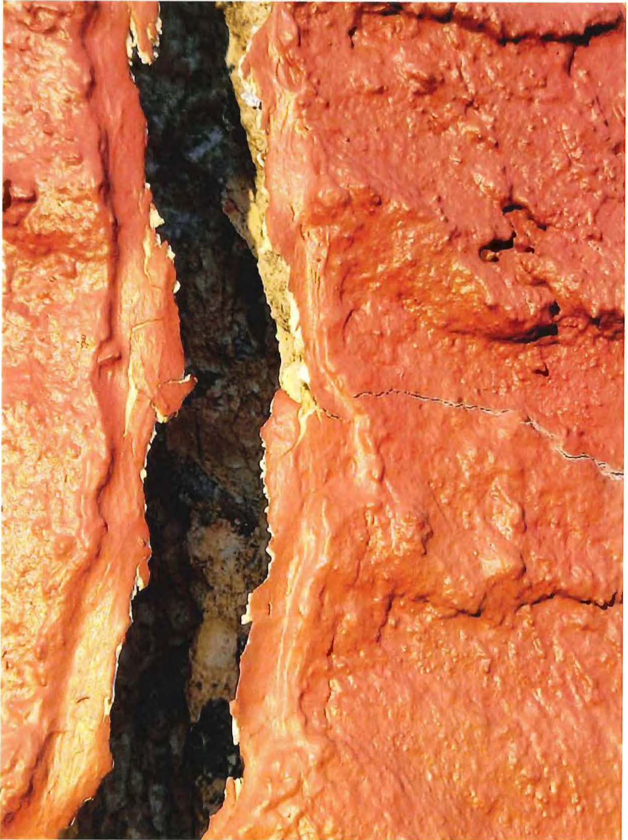
Inside South Wall Crack
