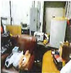
blocked electrical panel
