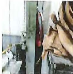
blocked fire extinguisher in shop
