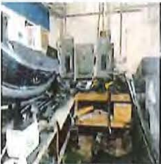
blocked electrical panels
