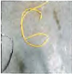
extension cord in bad shape in shop
