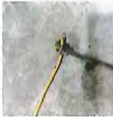
extension cord wired into the two ends of a service cord
